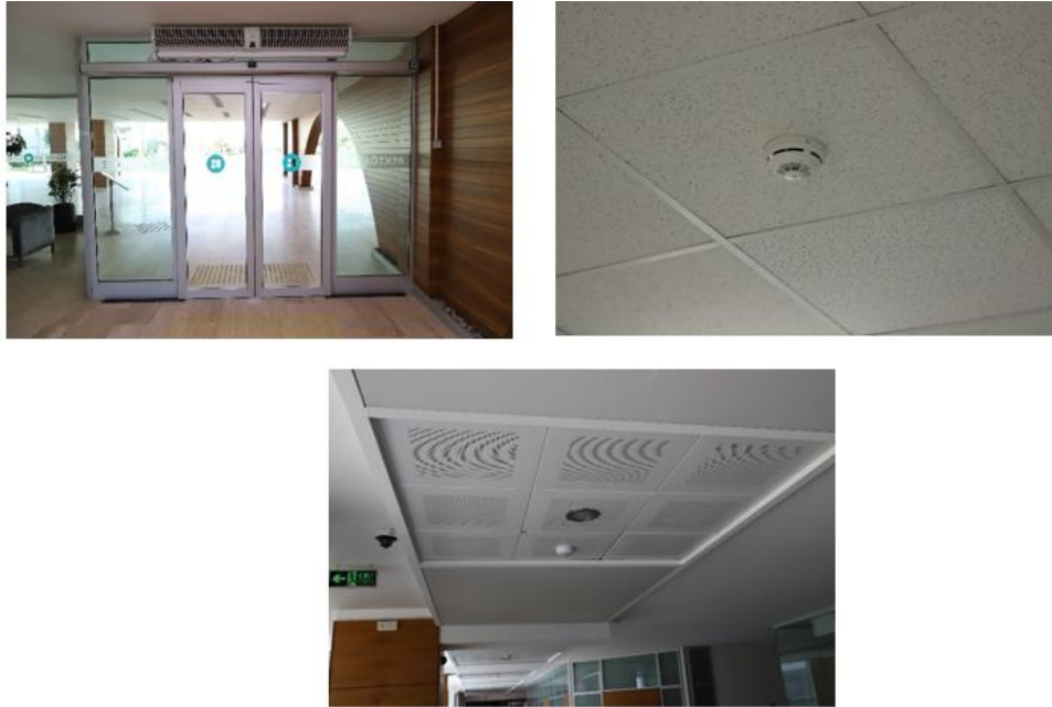
Figure 15: Smart Building implementation (Izmir Bakircay University, Turkey): The Automatic Door Sensor System; The Automatic Fire Alarm Sensor System
