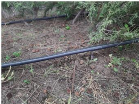
Figure 19a: Drip irrigation method
