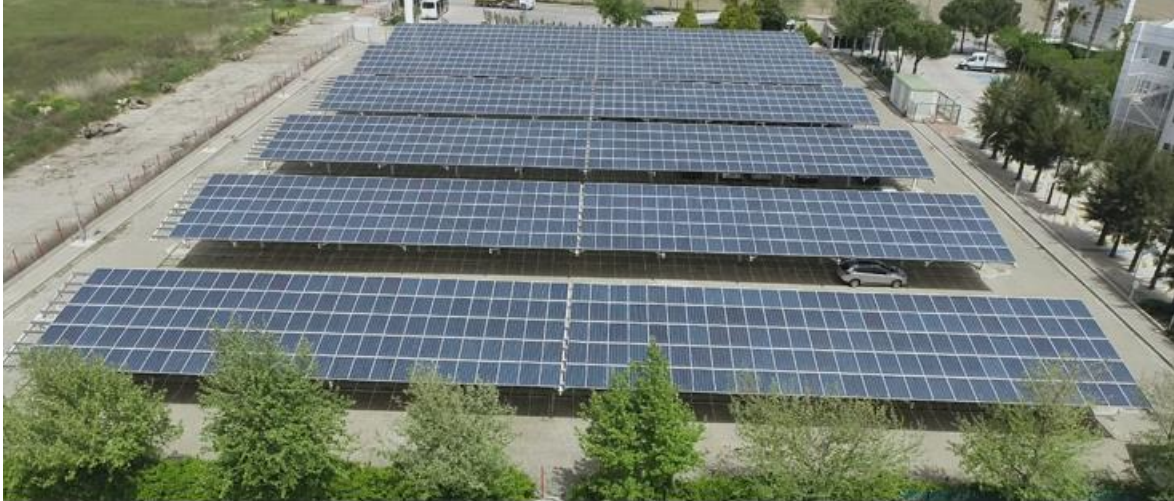
Figure 13: 400 kW PV Panels (roof of the personnel car park at İzmir Bakırçay University, Turkey)
